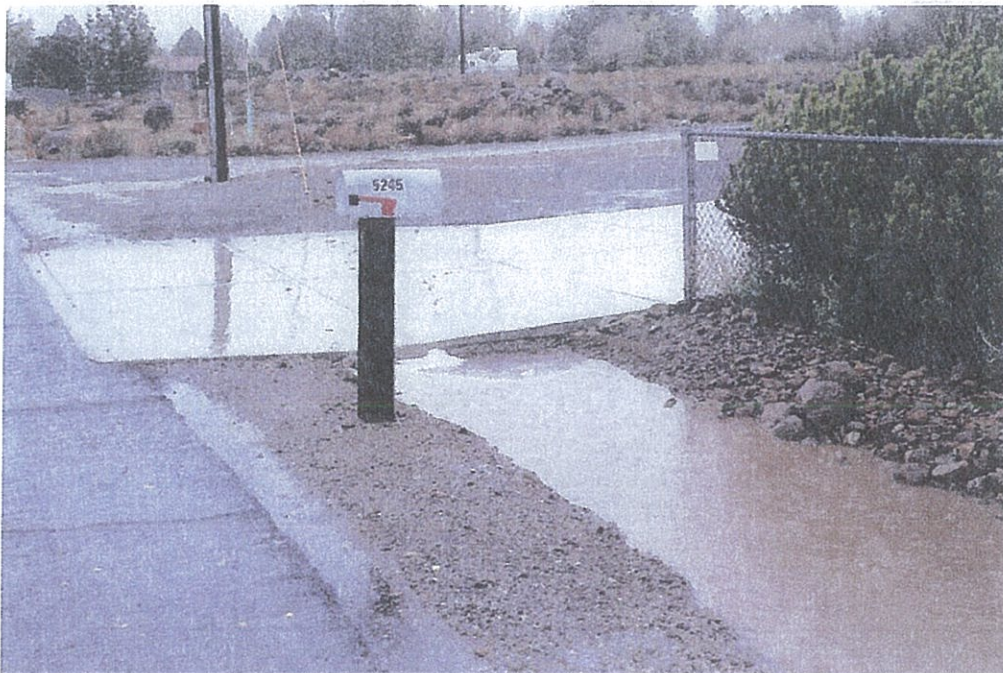
P8. Storm water Flow from the proposed Sierra Village on Shawna Lane. Note that this system is already at capacity. Discharge less than 2 cfs.
