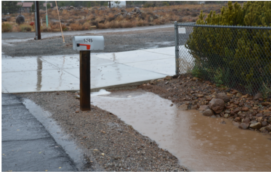
Ascente's floodwater under driveway on Shawna Lane
