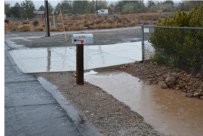
Photograph taken on October 16th, 2016 at 5:26 PM of 12" culvert on Shawna Lane. Note that discharge is at capacity for this storm water system.
